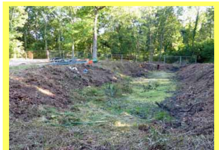
The site of Gennets Bridge Lock looking south in late September, following initial clearance. The compound will be to the left. The fencing running from left to right separates the Sussex Border path from the work site. (Photo: Dave Verrall)
